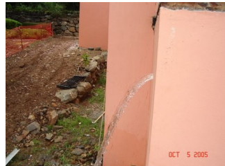
Water running out of wall
